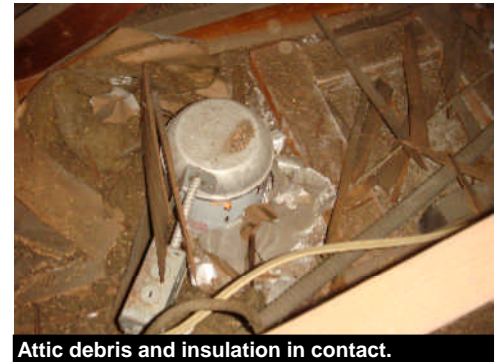
Attic debris and insulation in contact.
