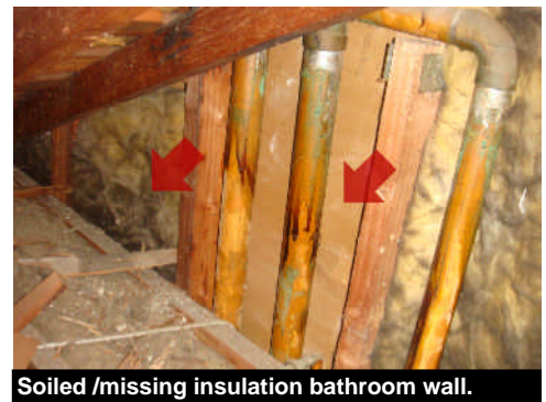
Soiled /missing insulation bathroom wall.
