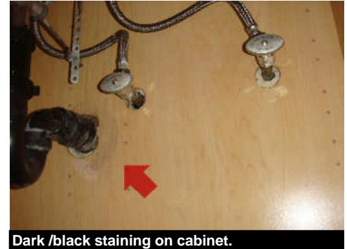
Dark /black staining on cabinet.
