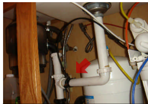
Improper saddle clamp on drain pipe.
