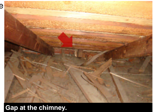
Gap at the chimney.
