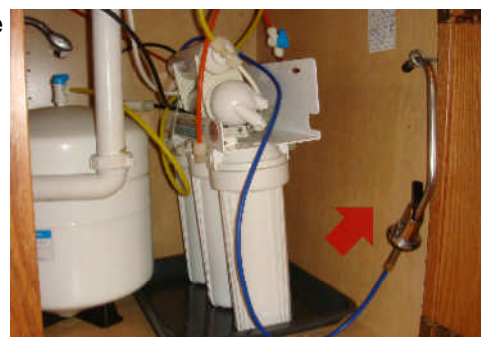
Irrigular location of filtered water spout
