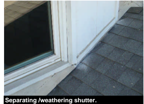
Separating /weathering shutter.
